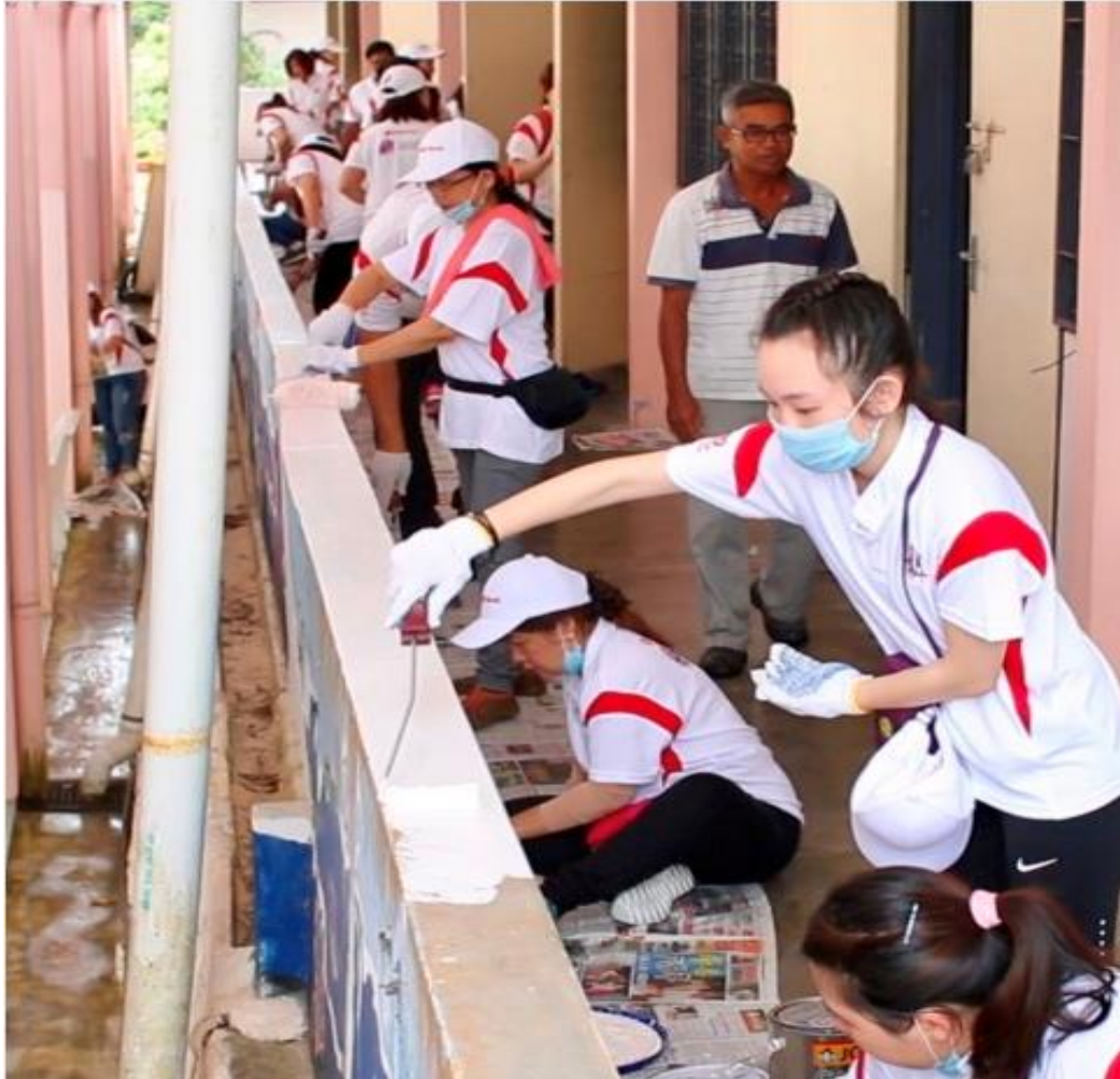
OCBC staff hard at work painting the corridor wall of the school
