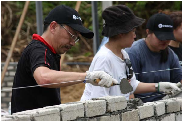
Mr Lim Khiang Tong, Head of Group Operations & Technology, OCBC Ltd (extreme left) laying bricks for the community hall.
